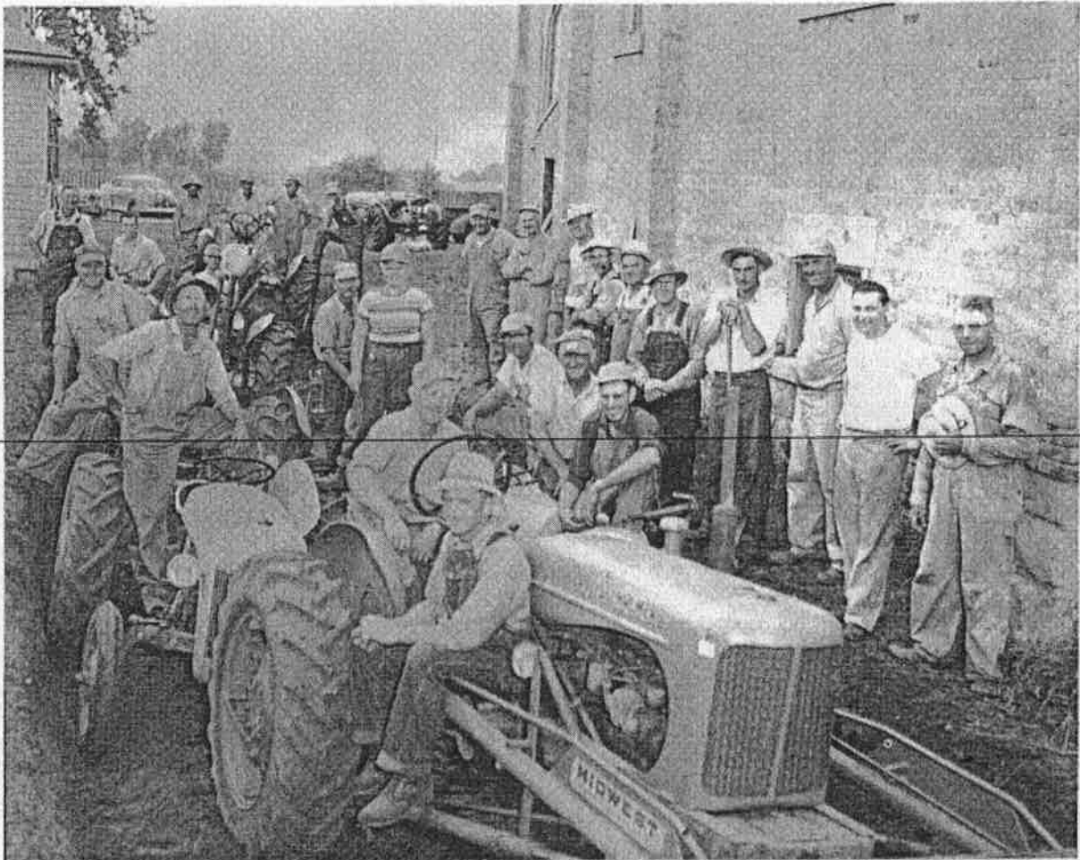
In 1954, this group of parishioners volunteered to dig a trench for the huge fuel storage tank, located between the rectory and the church. Rev. Ralph Muehlstein, pastor of St. Scholastica at the time, is pictured second from the right side. Others pictured include: Edwin Kimmet, Lambert Krocak, Mike Hinderscheid, Joe Hinderscheid, Elmer Studnicka, Eugene Jirak, John Hauer, Donnie Hauer, Francis Odenthal, Willie Odenthal, Frank Hinderscheid, John J. Prochaska, Otto Karcewski, Leonard Hruby, Erwin Schoenecker, Frank Ambroz, Bernard Ademmer, John Hinderscheid, Jim Kriha, John Kimmet, Louis Kriha, Ted Weiers, Roman Odenthal, and Louie Prochaska.
