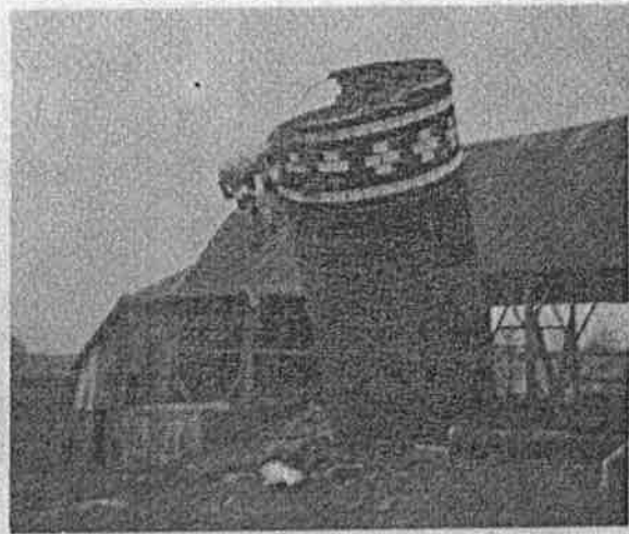
Barn and silo being dismantled. Note silo roof collapsing and falling to the ground. This was taken April 8, 1971. Helping Norbert on this project was Eugene Odenthal.
